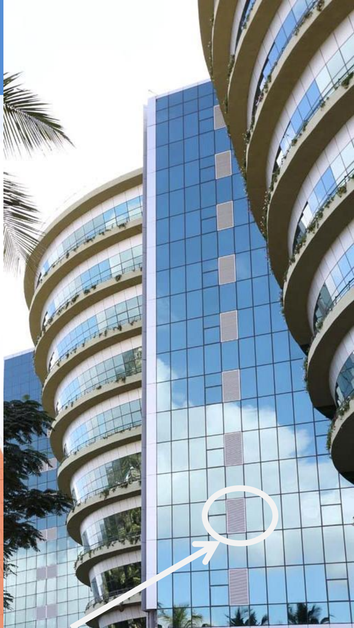
Exhaust grills with motorized dampers
